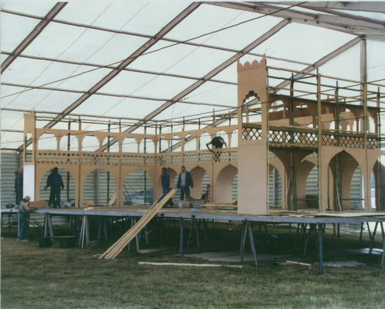
Indradyumna Swami (far left) carefully oversees the construction of Krishna's Village of Peace, including the elaborate stage (left).
