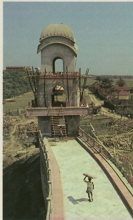
A worker carries cement along one of two wings that extend from the main structure. Between these wings is Śrīla Prabhupāda's “decorative pond.”
