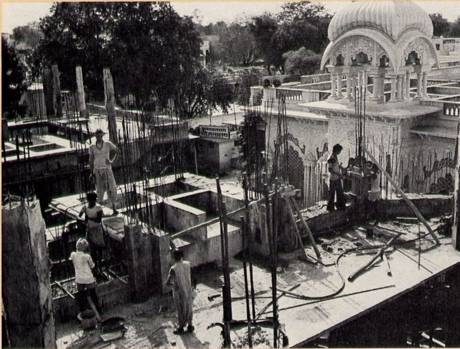
Support beams rise from the newly laid second story of the memorial shrine for Śrīla Prabhupāda in Vṛndāvana, India. The dome of the Kṛṣṇa-Balarāma temple appears at upper right.
